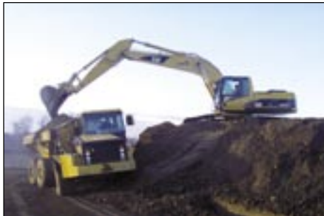
Apprentices learn to load haul trucks and the use of an excavator.
