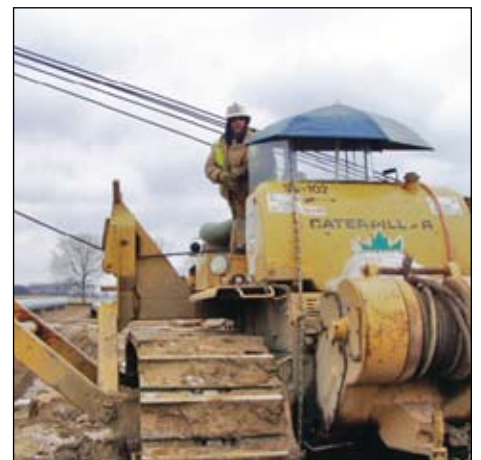
Mike Craft standing on the sideboom at the Rockies Express Pipeline job.
