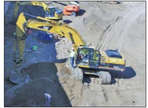
Mike Alderson working for The Simmons Co. at the new 34 story Marriott hotel in Indianapolis.
