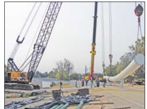
Tom Fronefield and Kirk Weeks lifting the beam for the walking bridge at IPFW.
