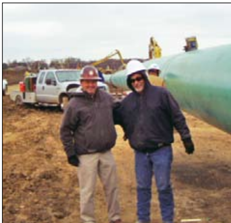
John Ballard and Bill King on site at the Rockies Express Pipeline.
