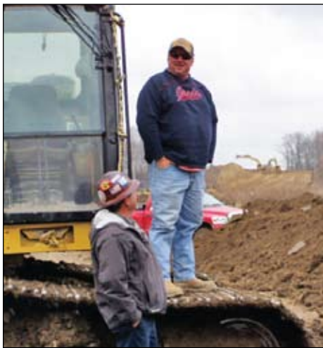
John Ballard and Scott Smalley at the Rockies Express Pipeline.
