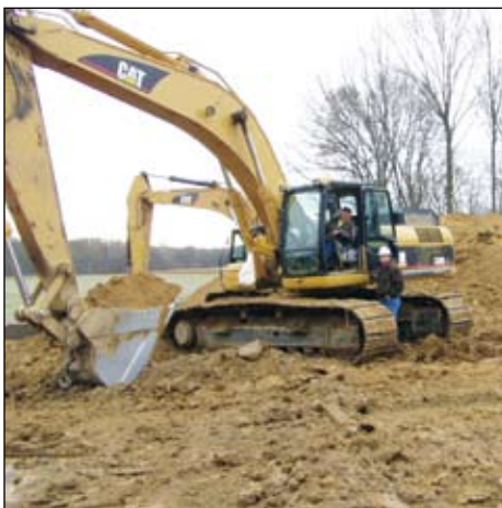
Frank Bowling operating an excavator and Brian Bramer at the Rockies Express Pipeline.
