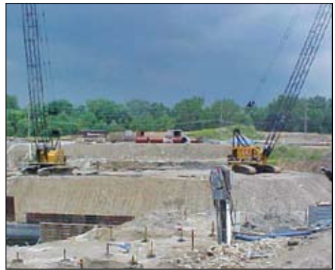
Bill Strasser and Jim Jones running the cranes at the WWTP for Hagerman Construction.
