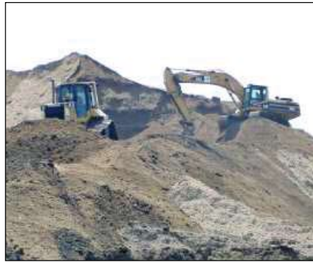
Steve Hardwick runs a bulldozer while Steve Tomlin operates an excavator at the new Colts Stadium.
