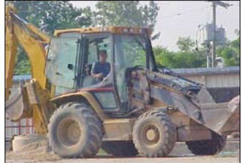
Robert Gallivan on his backhoe at the Ossian WWTP for Thieneman Construction.
