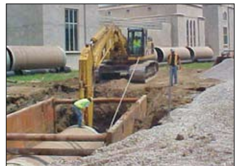
Kelly Shively digging with the excavator at the WWTP on Dwenger Ave. in Fort Wayne for Kreager Brothers.
