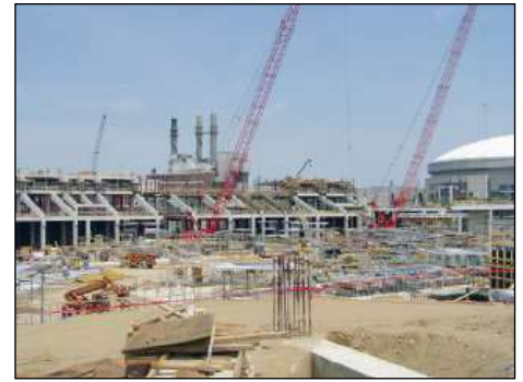
HIS, Maxim, Baker Concrete, and Hagerman are at the new Colts Stadium.
