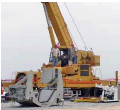
Chuck Boyle, David Miller and Shawn Hicks working for Midwest Mole on a 2,000 ft. bore under the runway at the Indianapolis Airport.
