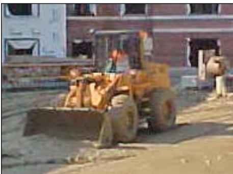
Scott Fernandes operating a front end loader for 3D Co. at the new Dormitory for Ball State.
