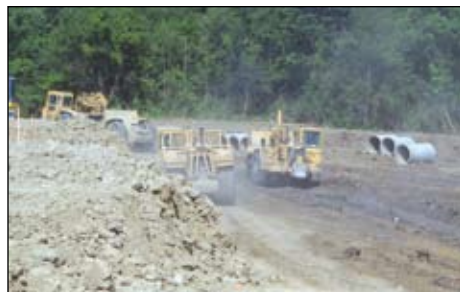
Cory Griffiths, Denny Johnson and Larry Wallace working for Gradex at the new Walmart in Fort Wayne.
