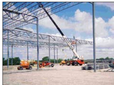
Bryan Maxwell setting steel for Sofco at the University loft in Hancock City.
