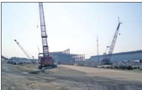
Lynn Jackson on the crane in front with John Chapman on the crane to the right working at SDI for Martin Inc.
