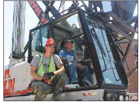
Lewis Troxell running the crane with apprentice Anthony Steinbrunner working for Ben Hur at Ball memorial Hospital.
