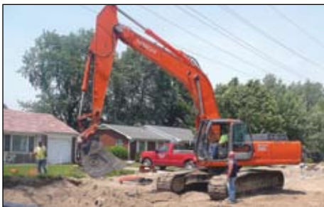
Jon Austin running the excavator for Atlas on Dixon Rd. in Kokomo.
