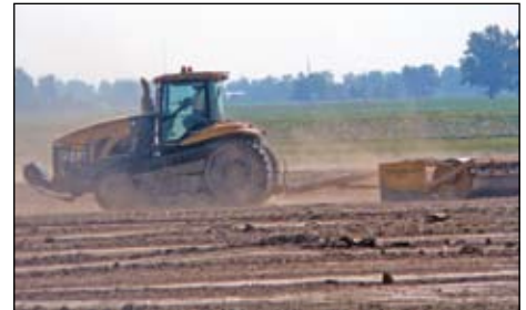
Jason Hurlock on a challenger at the Chrysler Project in Tipton working for Angelo Iafrate.
