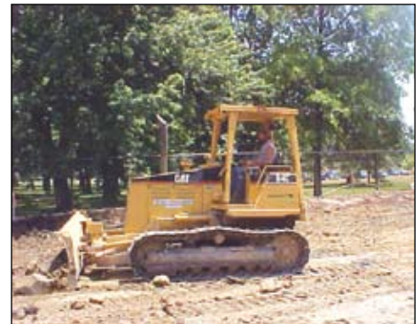
Lonnie Ailes working for Gale Tschuor running the bulldozer at Ball State.
