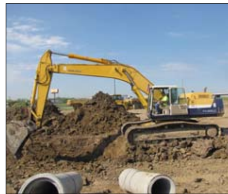
Randy Shipman running the excavator for Central Engineering at Mt. Comfort Rd. & I70.
